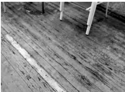
The old deck surface was in obvious disrepair and a safety hazard for the young military Brooks family expecting a new baby.
