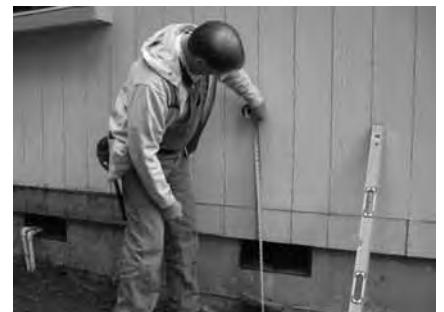
Measure twice, cut once was an adage Dave Delony stuck to during the new construction
